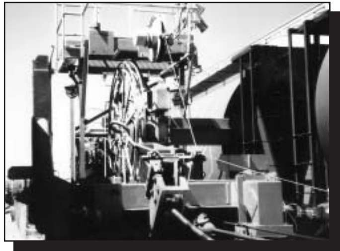
Tripper Conveyor To retrieve 600 feet of #4 AWG, 3 conductor, type G-GC, 600 volt cable.
