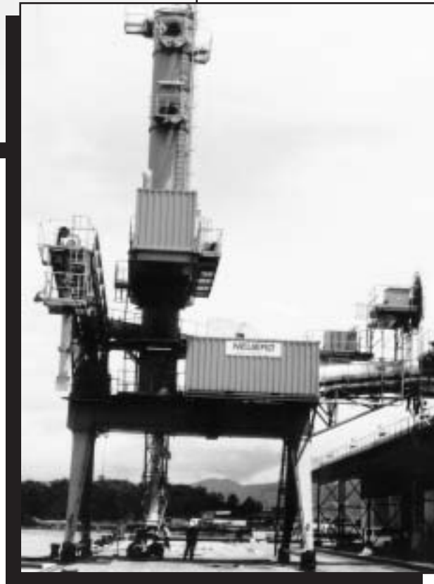
Ship Loader To retrieve 800 feet of #1/0 AWG, 3 conductor, SHD-GC-8 KV high voltage cable.
